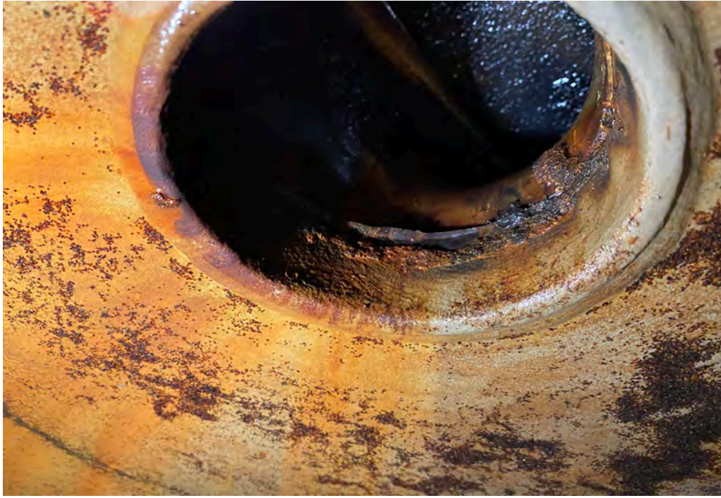
Bottom head nozzle N with corroded welds about the nozzle
