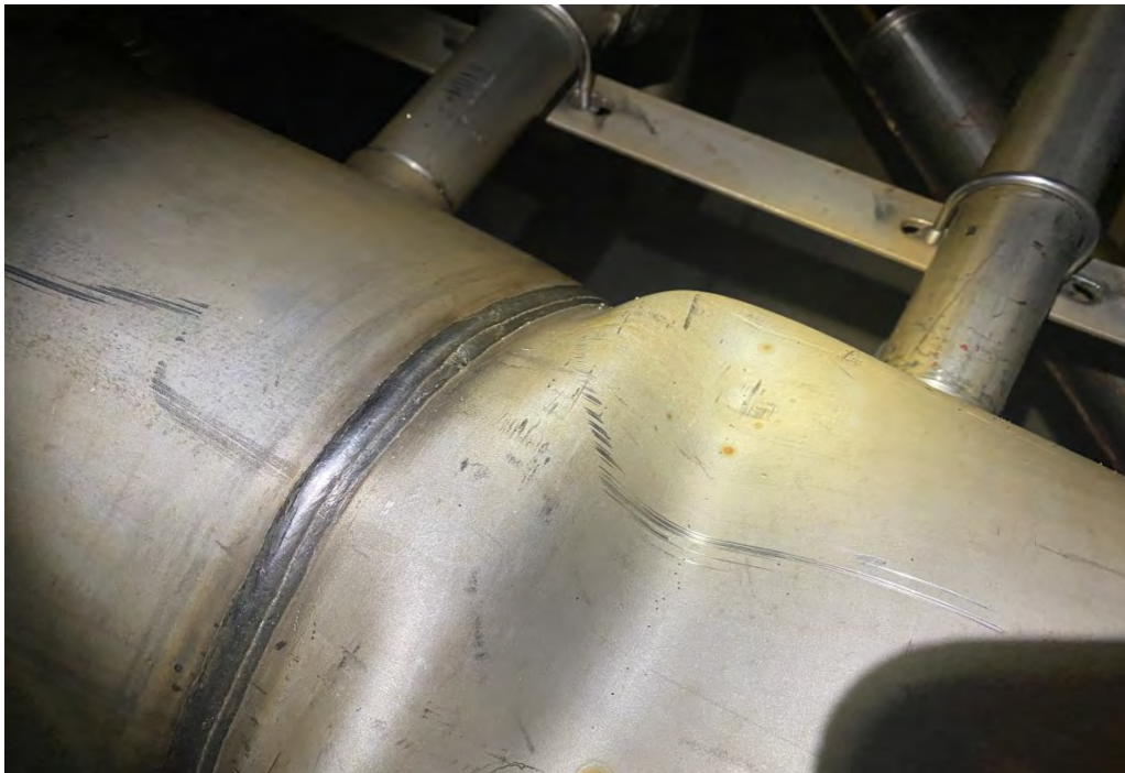
Header damage due to structural support failure
