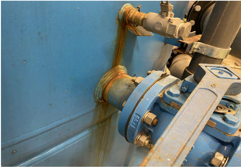
Threaded nozzle with signs of leaking
