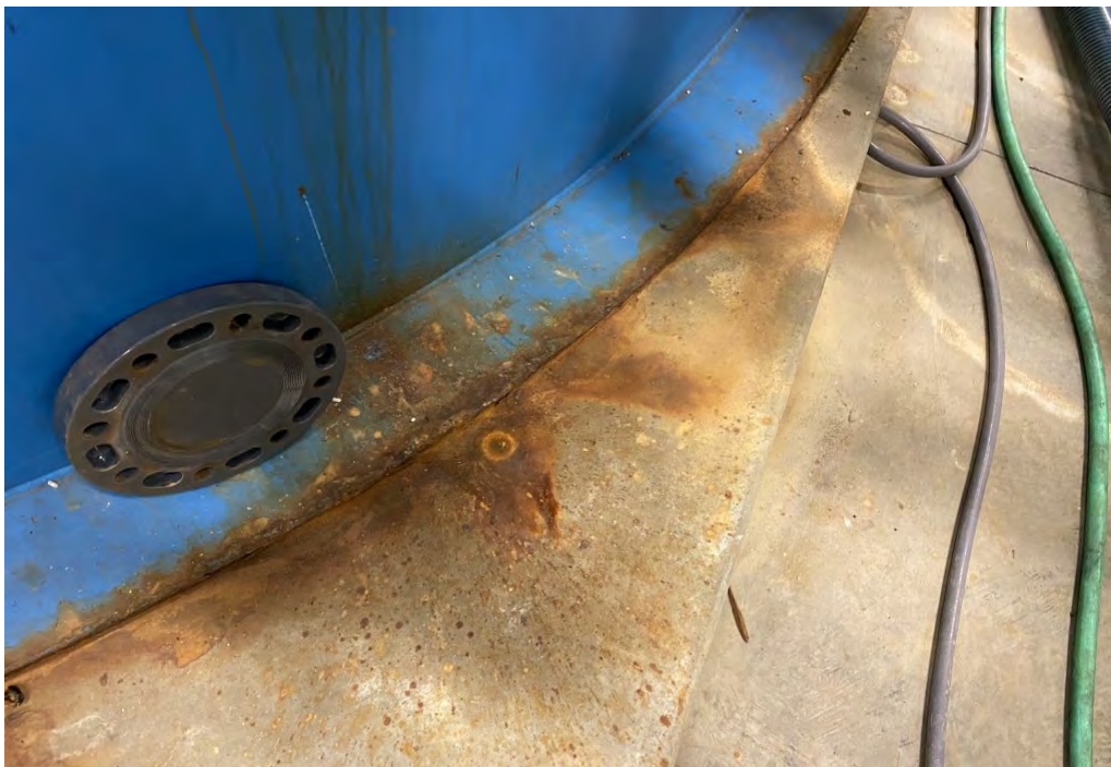
Vessel skirt chime with start of exfoliation corrosion
