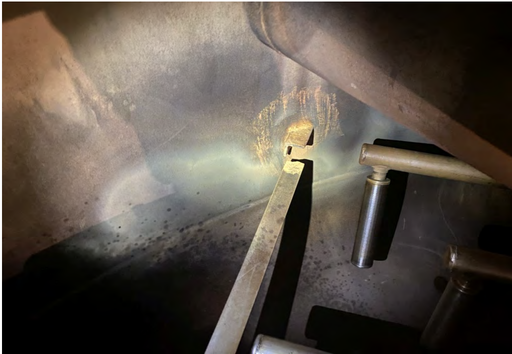
Lower BOM piping support failure
