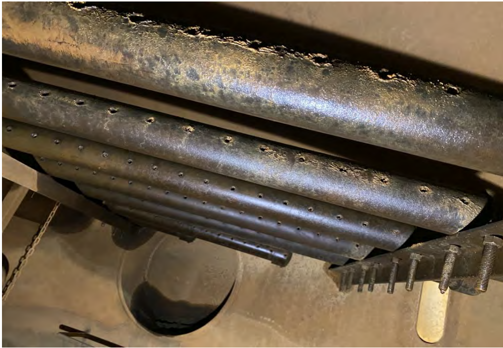
Internal upper BOM piping
