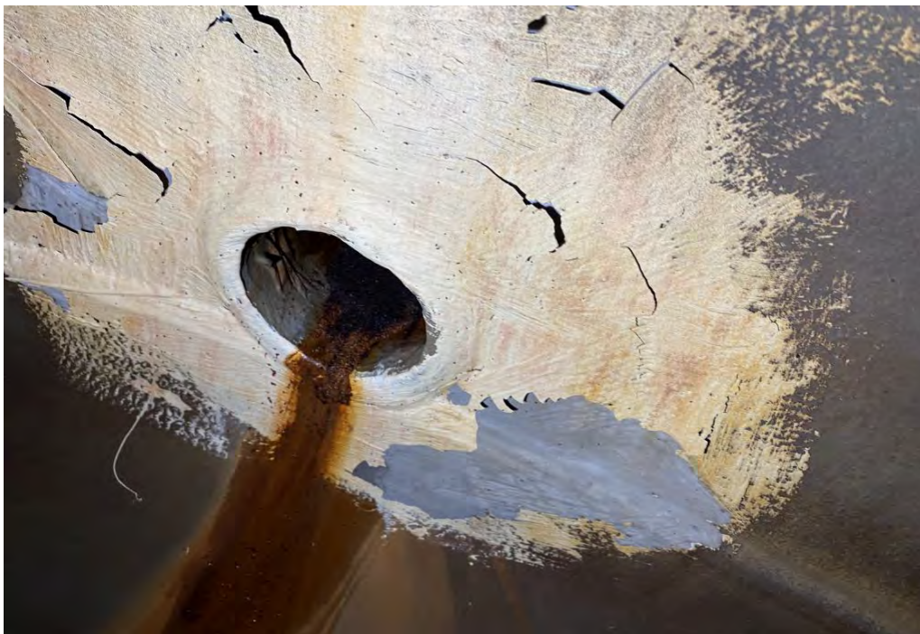
Internal lining disbonding
