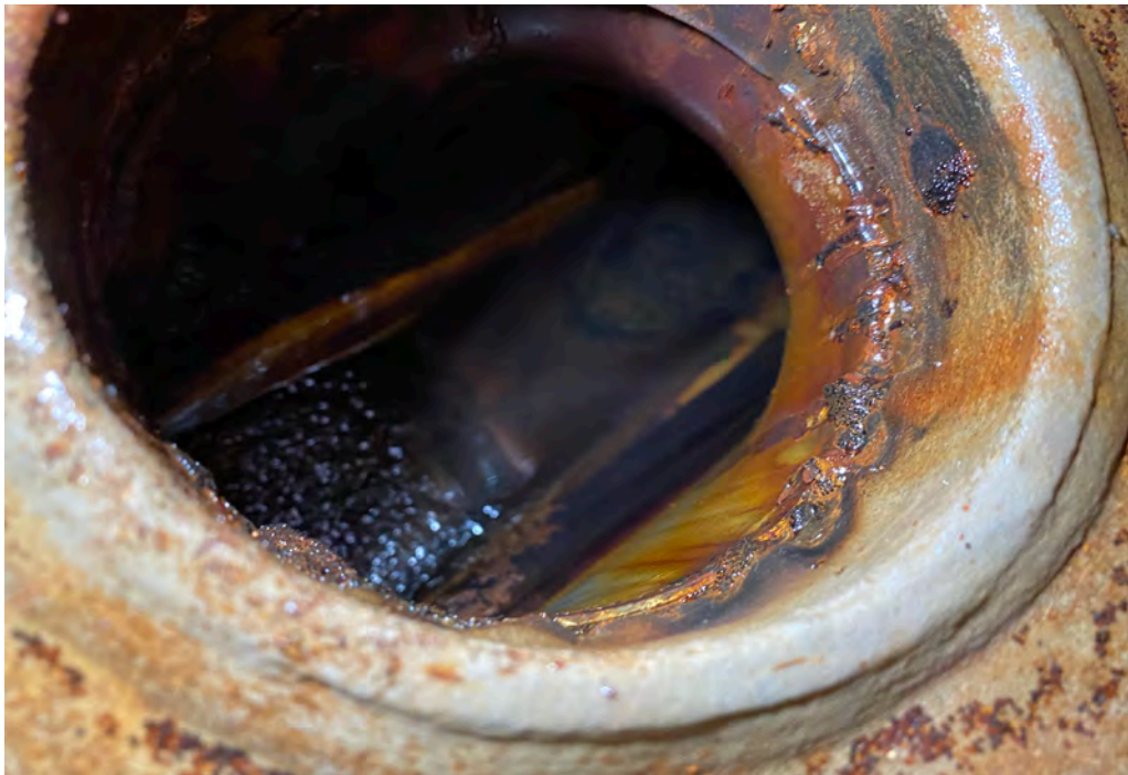
Nozzle N with corroded welds about the nozzle
