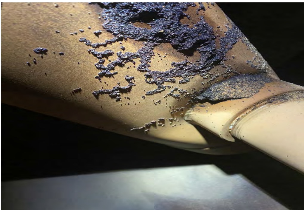
Lower BOM damage to header from support failure
